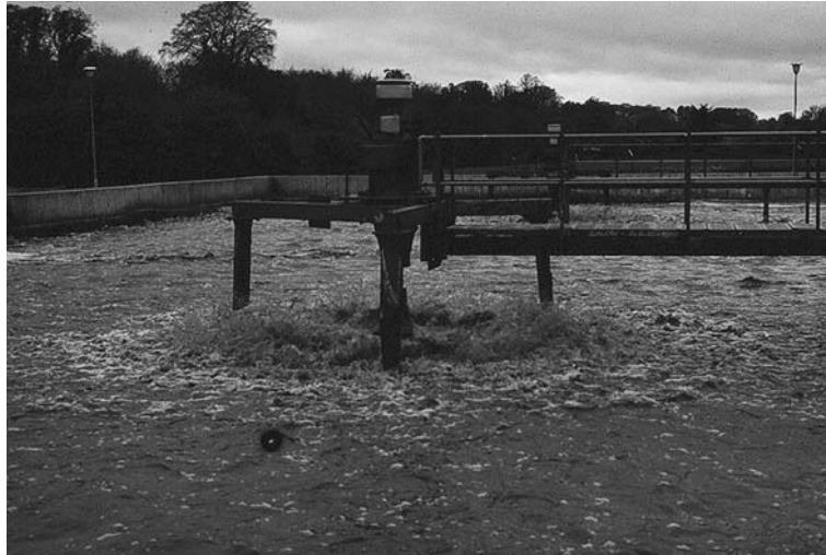
FIGURE 17.5 A fixed vertical aerator creating both aeration and mixing within the aeration basin.
