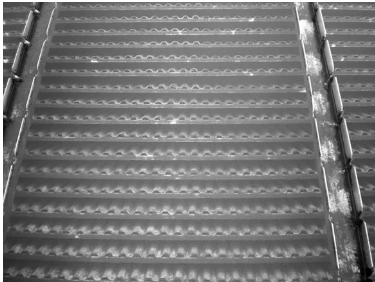
FIGURE 10.7 Inclined lamellar plates placed near the surface of upflow clarifiers enhance solids removal efficiency.
