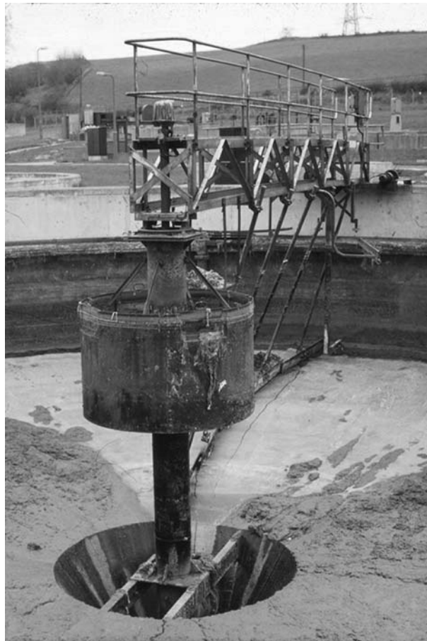
FIGURE 14.12 Radial flow tank showing inlet, diffusion box, scraper blade, support column, sludge sump and scum board.
