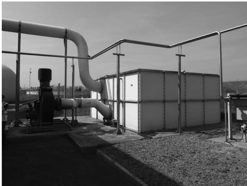
FIGURE 20.12 Air is vented from covered tanks and enclosed areas by large fans and is passed through activated carbon filters to remove odours. This filter is filled with mussel shells on which bacteria develop. The filter removes odours by bacterial adsorption and subsequent oxidation, while the calcium in the shells neutralizes any acidity.
